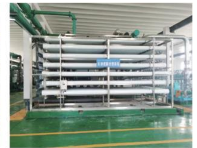
14400T/D Energy Equipment Company in Sichuan
