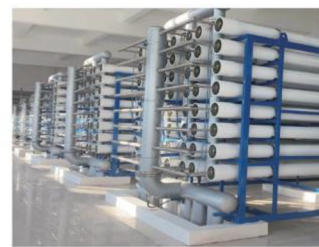
50000T/D Water Treatment Company in Cangzhou
