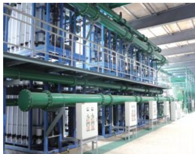
28800T/D Thermal power company in Shandong - make-up water treatment and zero-discharge project
