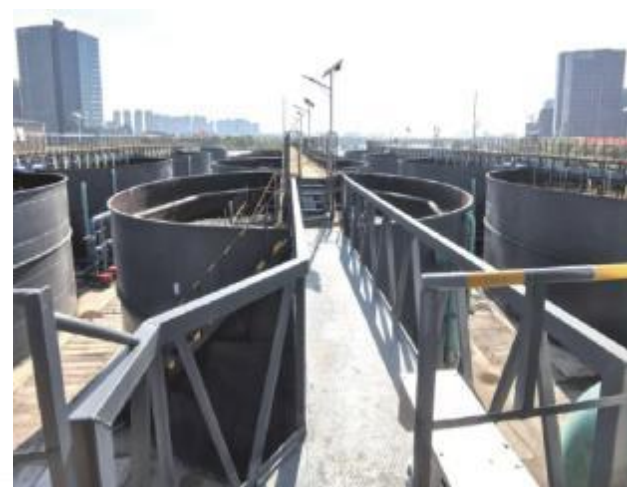
40000T/D Municipal Sewage Plant in Nanjing
