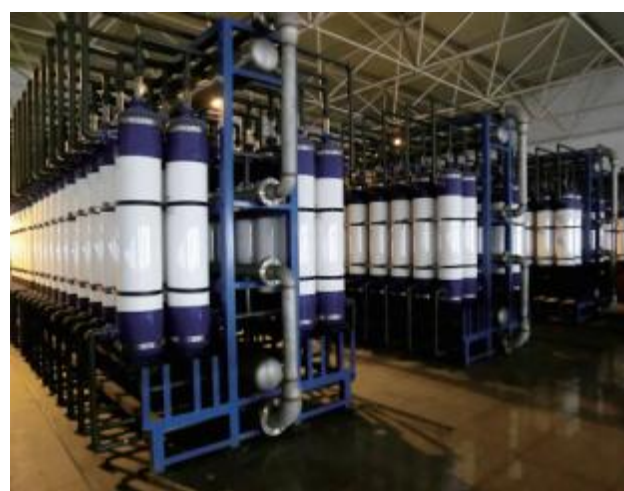
500000T/D Power company in Shandong - Boiler make-up water treatment project
