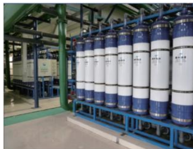
4900T/D Seawater Desalination Project in Shandong
