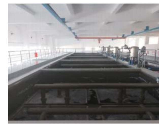
5000T/D A sewage treatment plant in Inner Mongolia
