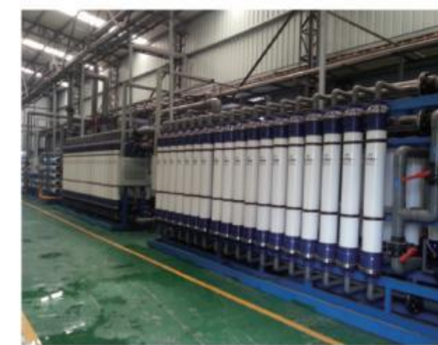
50000T/D Water Treatment Company in Cangzhou
