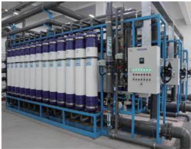
20000T/D Water Plant Upgrading in Shandong
